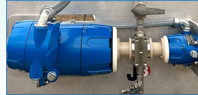
Pictured above: The proprietary Gen3 prototype spectrometer installed on an Eagleford wellsite
