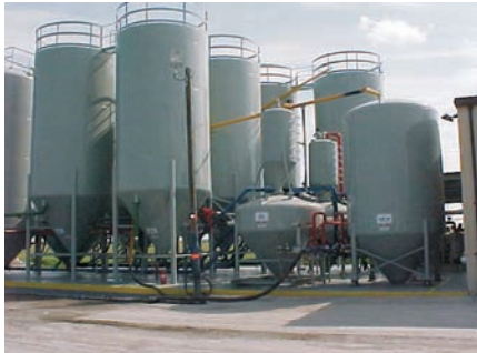
Vacuum/Pressure Plant Cisco, TX
