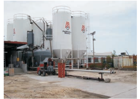
Vacuum/Pressure Plant Cuidad del Carmen, Mexico
