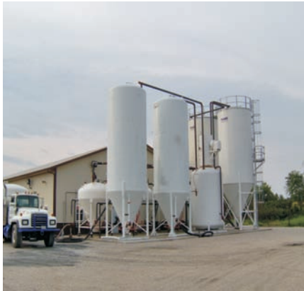
Vacuum/Pressure Plant Lawrenceville, IL
