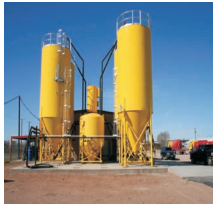
Vacuum/Pressure Plant Odessa, TX
